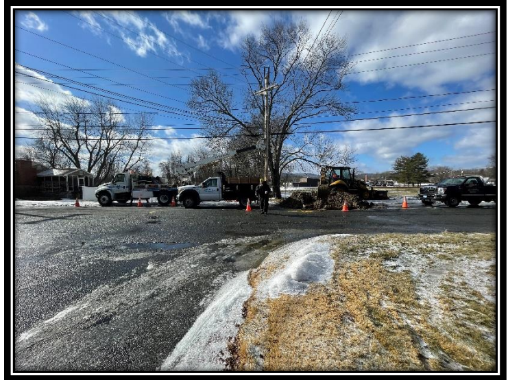
Water Main Break on Parkview Drive
